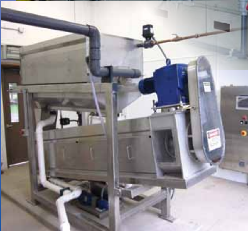
DSP Screw Press, Groton, NY WWTP
