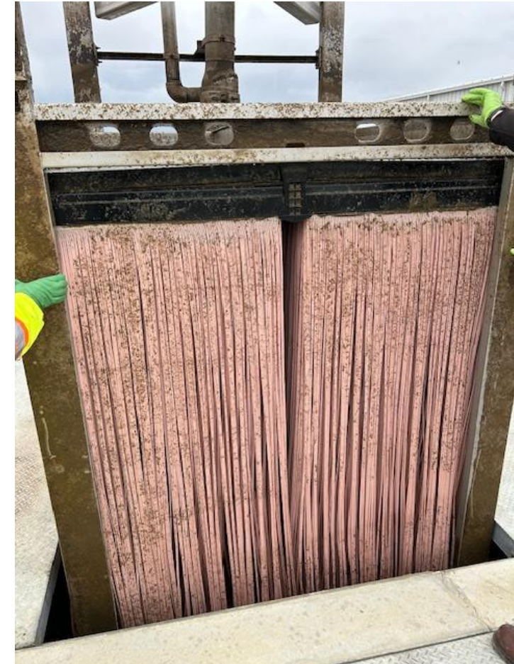
6-month membrane cassette inspection
