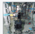
Ozone Injection Skid
