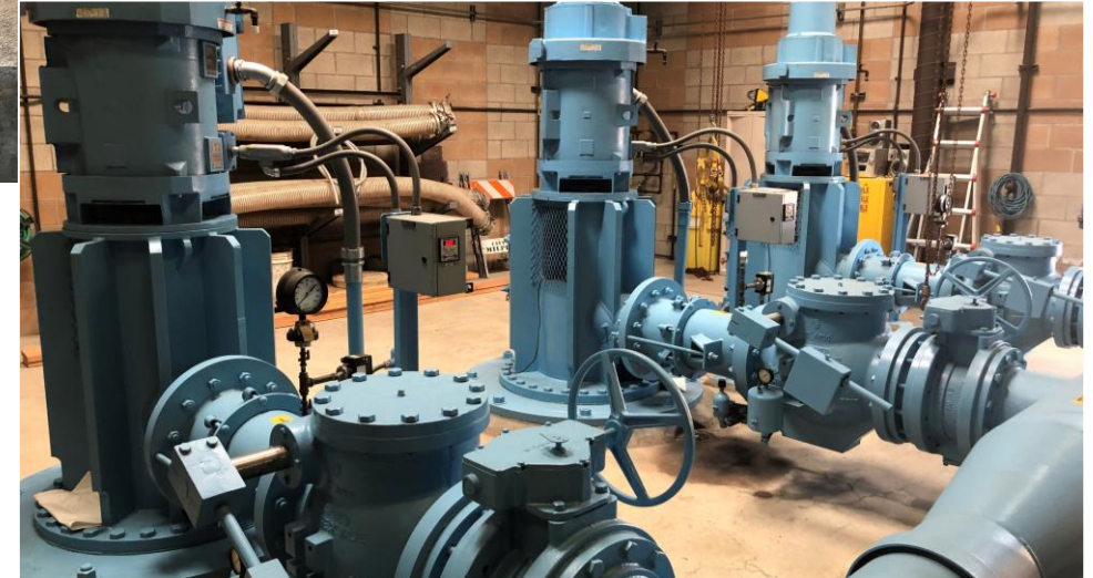
Milpitas Ayer Reservoir & Pump Station
