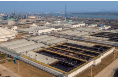
Industrial wastewater treatment facility Lianyungang, Jiangsu, China
