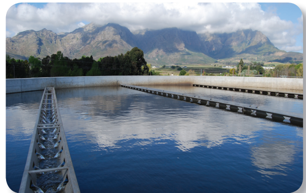
Treated effluent produced from an AquaNereda® reactor.
