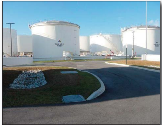
Commercial Aviation Fueling System - Fuel Storage Tanks
