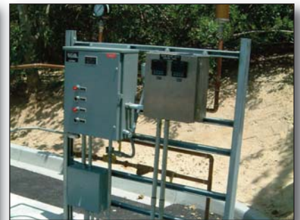
Remote SCADA control
