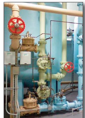
Multiple Valves in Industrial Application
