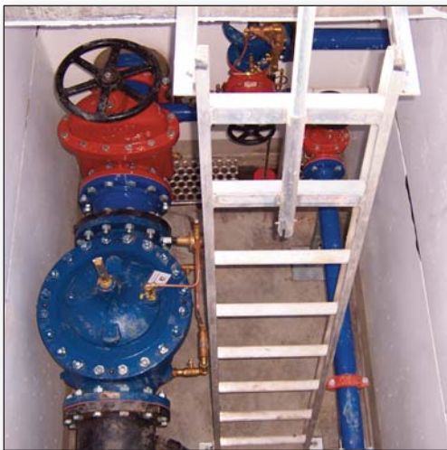
Pressure Reducing Station in a municipal water distribution system
