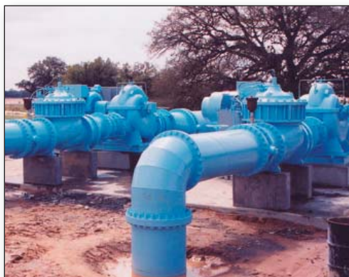
30-Inch Pump Control Valves
